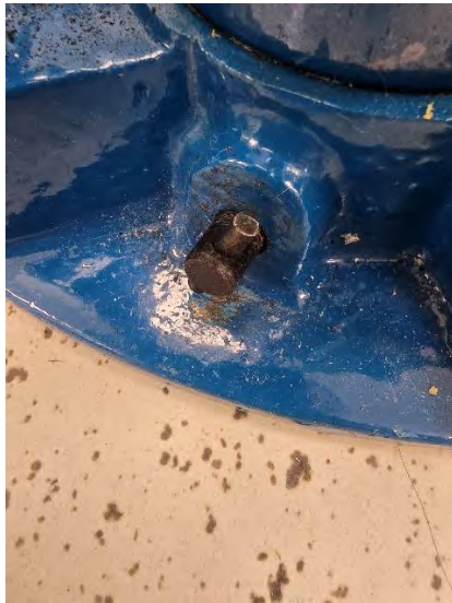
Figure 289: Closeup of Release Valve
