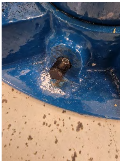
Figure 282: Closeup of Release Valve
