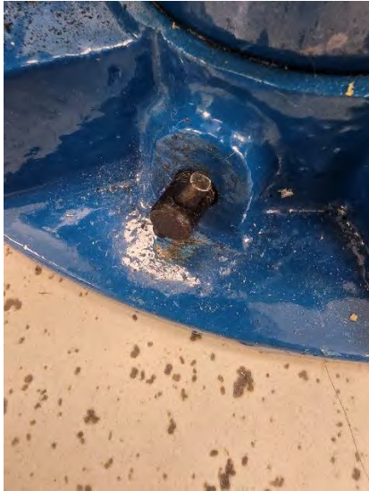
Figure 275: Closeup of Release Valve
