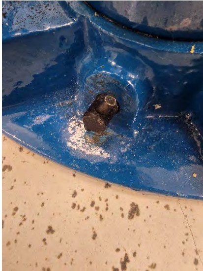
Figure 282: Closeup of Release Valve
